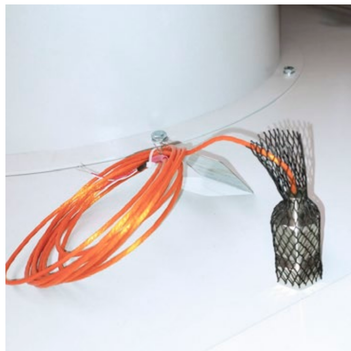
Fire Suppression System
